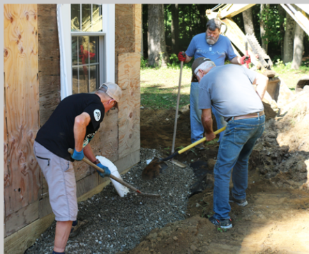
Greg Durgin, Larry Dunn and Jim Tukey spread crushed stone around new perimeter drain pipe installed with help of BA Perry Earthworks.
