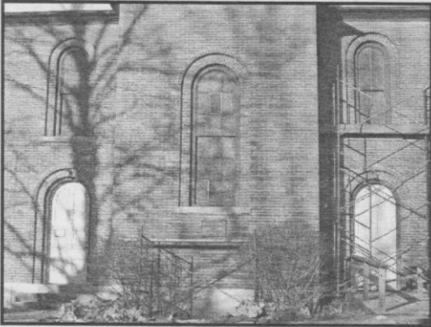
A grant from the National Trust for Historic Preservation allowed the UMH to install UV-resistant Plexiglas over five delicate windows including these three on the façade.
