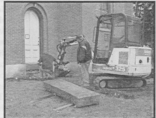
Re-grading the lot was the perfect opportunity to switch the broken left front step with the right one. The crack is now hidden under the handicapped ramp.
