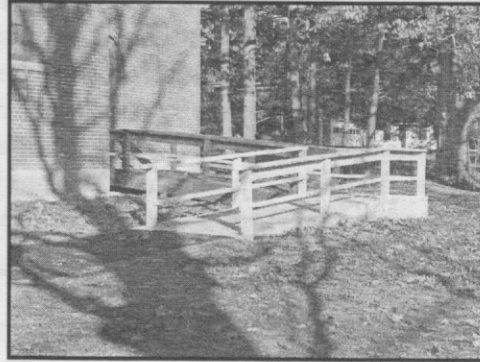
Changing the contours of the lot resulted in earth being taken away from several areas. This required an extension of the handicapped ramp which was done by James & Wheeler, local contractors.
