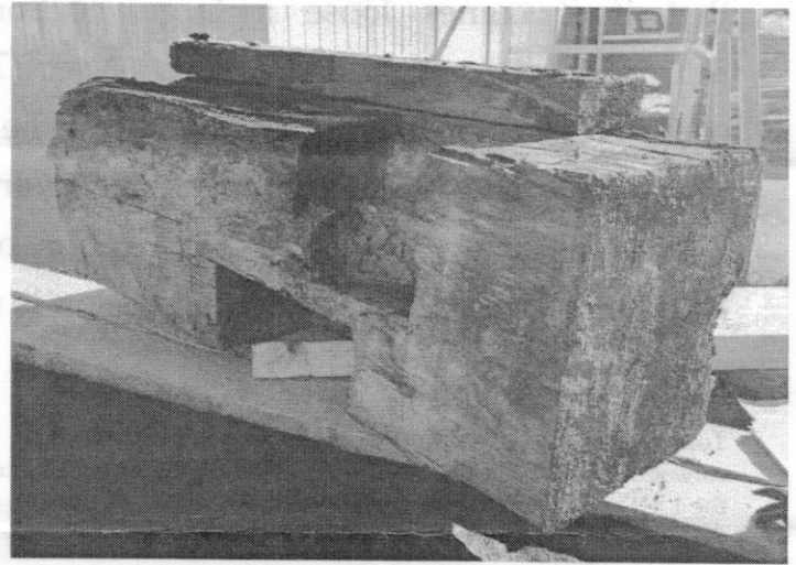
This short section of the original narthex beam will be saved since it shows the deterioration caused by 89 years of dampness and also documents the special "dovetail" that links the beams together. It will be replicated in the new timbers. (J. Perry photo)
