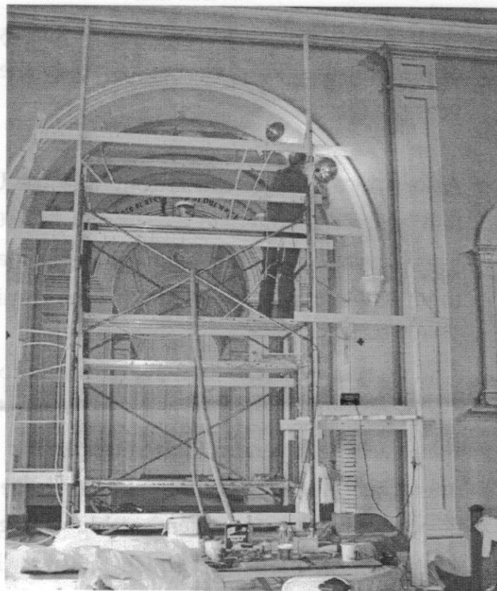
Tony Castro erected scaffolding in the arch to the so he could consolidate loose plaster, re-adhere it, and fill the numerous cracks that developed when the arch began to fail. In this photo he is in the 1 o'clock position with his light doing some in-filling. The final application of colors will take place in the spring. (Péladeau photo)
